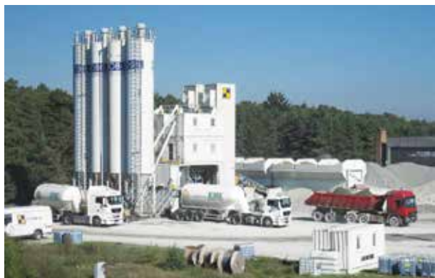
Fig. 7. An example of concrete-mixing plant for road construction
